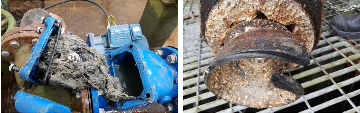
Figure 112 – Pictures of issues identified by the Proactive Analytics Centre: the image on the left demonstrates the impact of wet wipes clogging a non-return valve, while the right shows fat, oil and grease stuck to the pump impeller and reducing efficiency
