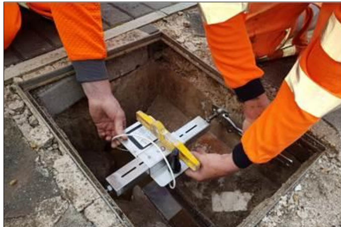
Figure 134 – Low-cost sewer sensor being installed
